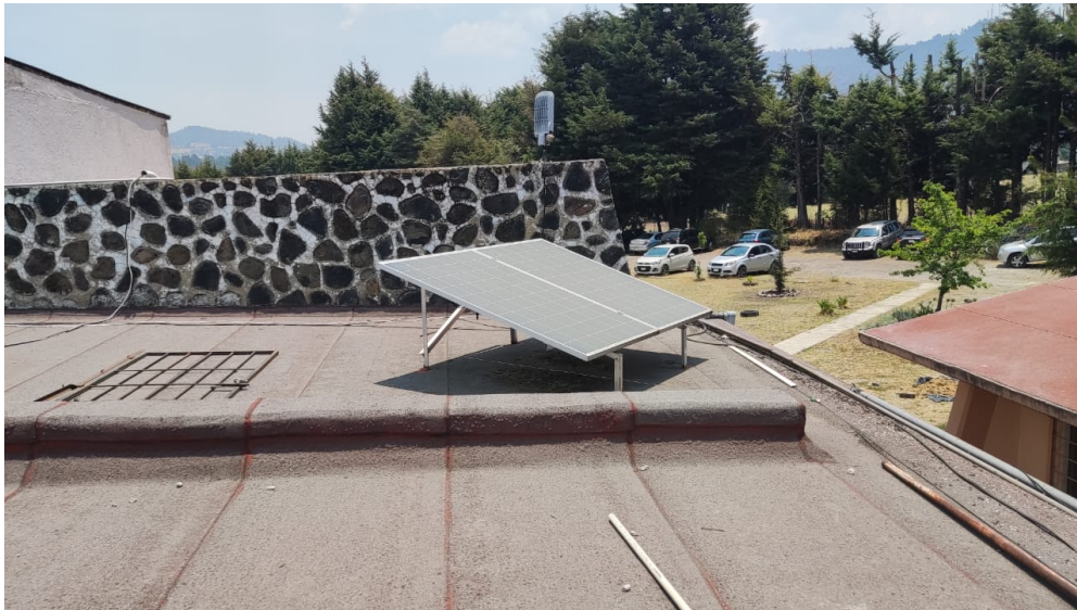
Figura 3.5 (a) Panel solar instalado
