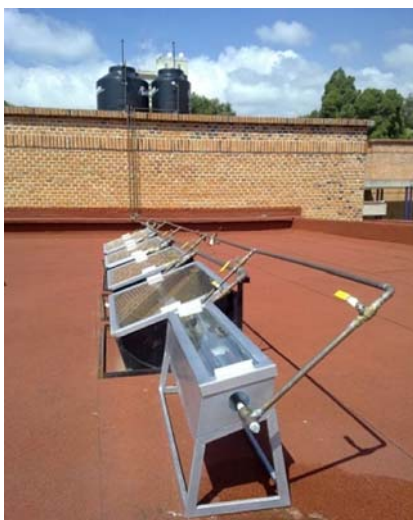
Fig. 7. Overview CIICAp rooftop concentrators, power piping and tank and receiving tank.
